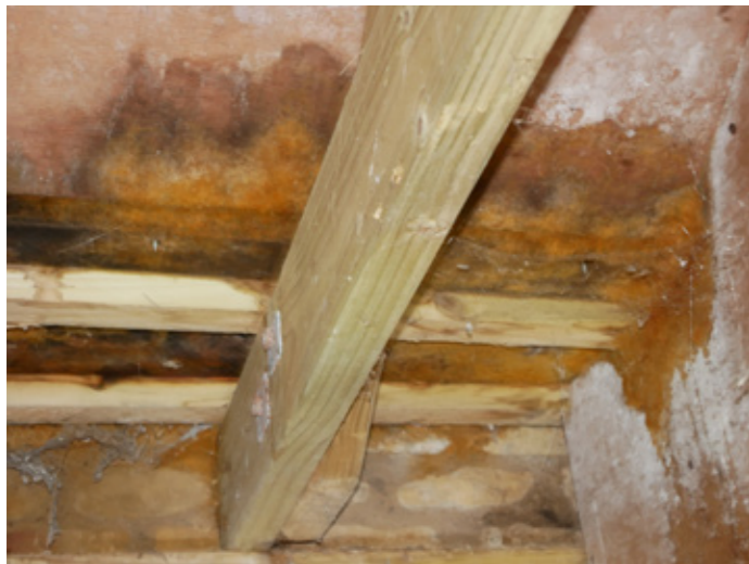
P45 Byre interior damp damage detail
