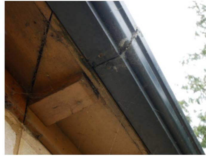
P39 Cedar Centre leaking gutter
