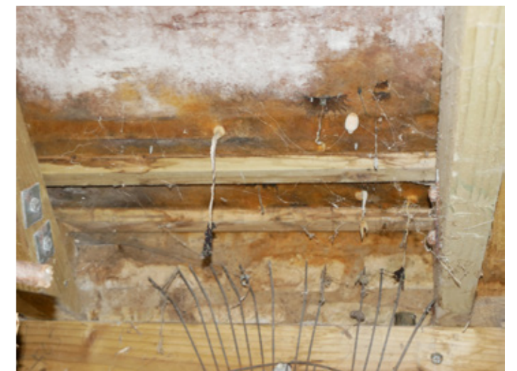
P44 Byre interior damp damage fungus
