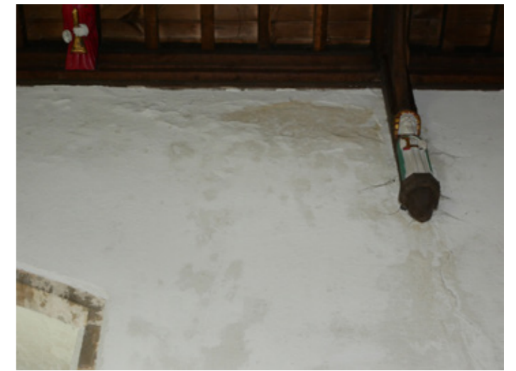
P32 North Aisle North wall damp damage
