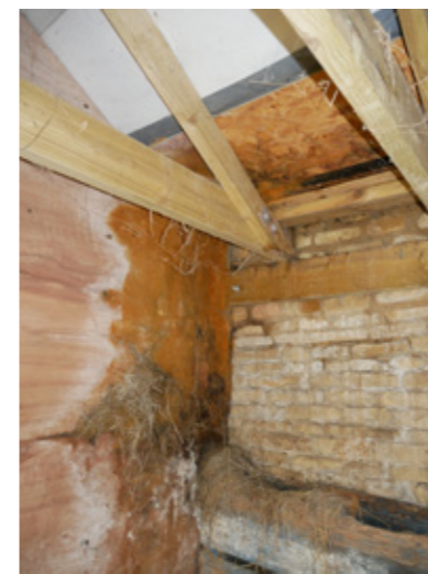
P43 Byre interior damp damage
