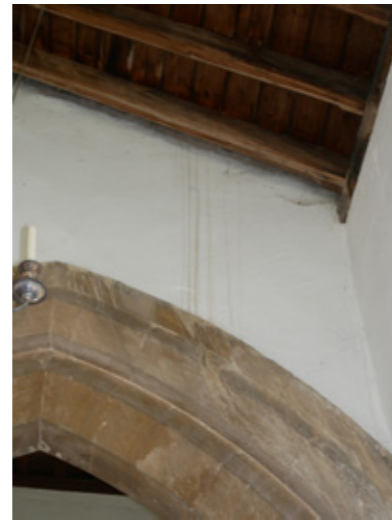
P30 Vestry North wall water streaking
