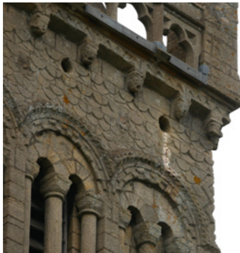
P09 Tower East elevation bird mess
